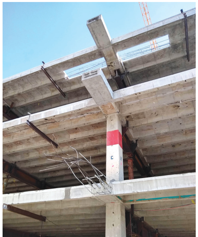
Figure 4. New cantilevered girder ends at various stages of construction, with continuous shoring installed.
